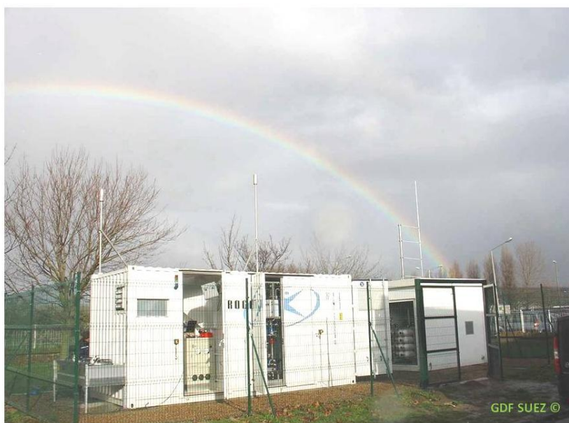
Figure 2 - The two containers of the Hythane® station.
